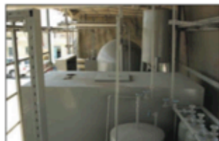
Interior view of fermentor, media tank, water supply tanks, and gas cylinders connected by pipes.
