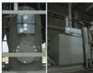
Fermentor. Exhaust gas compressor.
